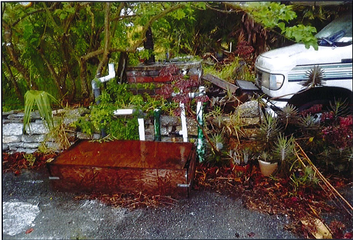
Photograph No. 19 View to the to the north of a potential irrigation well on the central-western portion of the Subject Property.
